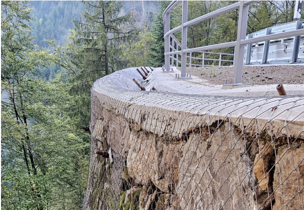
Figure 6. Retaining wall on a bend on the L126 between Oberried and Notschrei. At the top right, you can see the vehicle restraint system and, directly adjacent to it, the road surface, which is treated with de-icing salt in winter.
