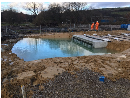
Figure 9. Photos of the box culvert after the dewatering system was turned off.
