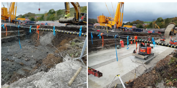
Figure 8. Photos of the construction works from left to right: (a) excavation in dry ground, (b) laying the culvert foundation.
