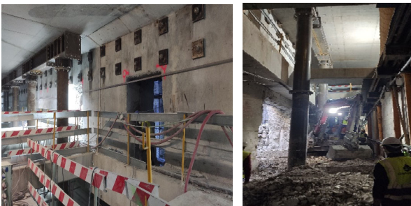
Figure 10. View of one of the openings, prestressed bars (first stage) and the temporary steel portal (second stage).
