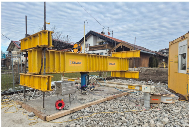
Figure 1. Test Pile Setup: Recorded driving time per meter (top), schematic representation of DFOS arrangement along the pile (middle) and practical realization of test rig (bottom)
