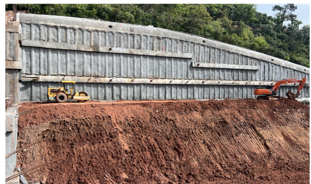
Figure 10. View of the final stage of earth fill execution, implemented as the first reinforcement measure at East side wall.
