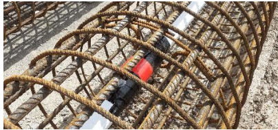
Figure 12. Monitoring devices installed: inclinometers installed inside the bored pile wall.
