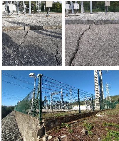
Figure 5. Existing pathologies at the substation.
