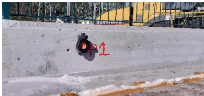
Figure 11. Monitoring devices installed: topographic targets installed in the reinforced concrete wall.
