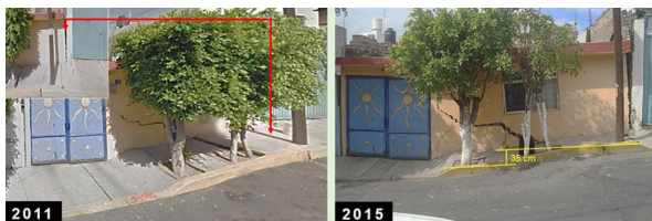
Figure 2. Damage and magnitude of a step crack in Iztapalapa. (Auvinet, et al., 2020)
