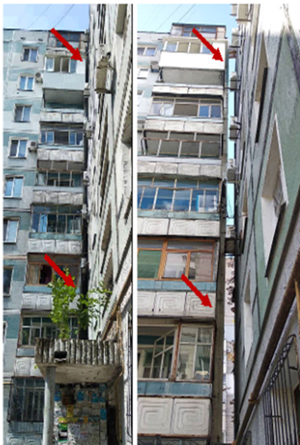
Figure 9. General view of the expansion joint between the block sections No. 3 and No. 1 at 23 and 25 Preobrazhenska St. in the city of Zaporizhzhia before and after leveling.
