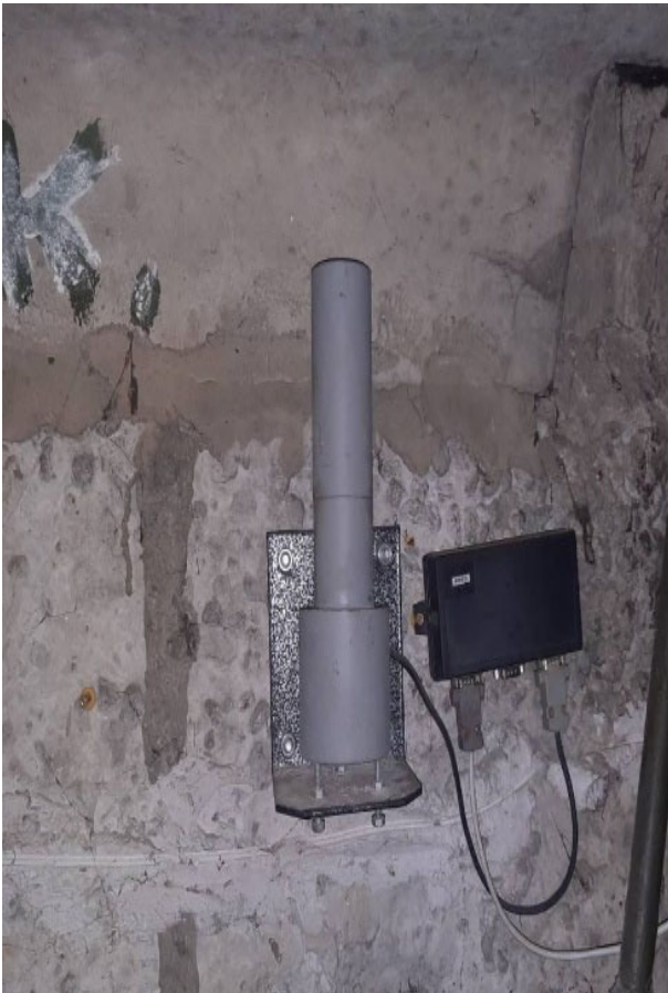
Figure 3. The appearance of the universal inductive device sensor installed on a wall in the basement of the building.
