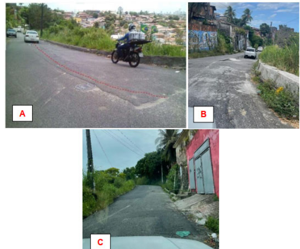
Figure 9. History of the Crack in the Study Slope.
