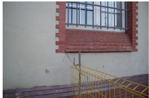
Figure 9. Characteristic pattern of damage to the building walls near the excavation
