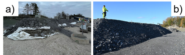
Figure 4. Construction of the protection layer with crushed limestone. a) during construction, and b) after completion. Photos from NOAH and NGL.
