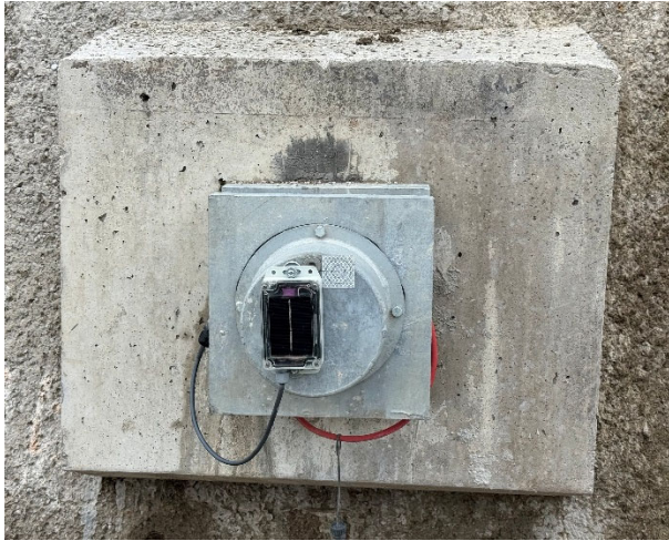
Figure 3. Cellular Solar Panel for a grid-independent data-transfer solution
