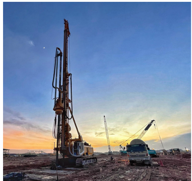
Figure 8. Installation of the FDC columns with a maximal length of 27 m using a BG28 with Kelly extension
