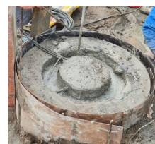
Figure 8. Grout with high strength concrete between steel pipe in the middle and spun pile
