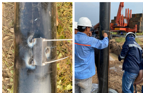
Figure 7. Cable attachment during steel pipe insertion into hollow part of the spun pile
