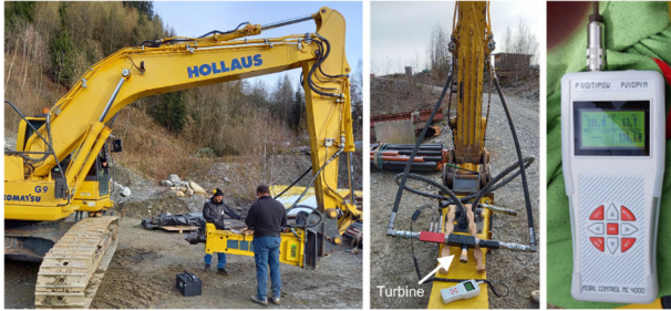
Figure 4. Test Zillertal: Measurements of oil flowrate before driving.
