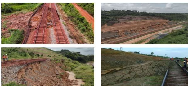
Figure 1. Examples of slope instabilities observed along the Carajás Railway in Northeastern Amazon – Brazil (Futai et al., 2024).
