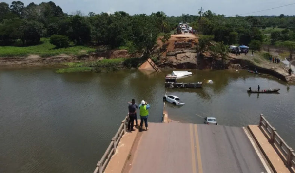
Figure 4. Total collapse of a bridge in BR 319 road, near Manaus city, Brazil (Globo, 2022).
