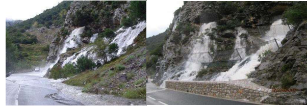
Figure 30. Safety problems due to falling stones and hydroplaning on the N-621 road after heavy rain. Situation PK 158.140 MI produced by the heavy rains on the rocky slope where the work was carried out.
