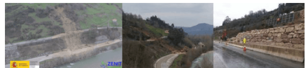
Figure 24. Landslide caused by heavy rains, causing the total cut of the N-623 and N-623a road in the afternoon of 10 March 2016. PK 117+300 left bank
