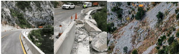
Figure 14b. This is the conference logo. Situation at KP 160.700 MD caused by heavy rains after cleaning the remains of stones from the roadway and placement of material by helicopter.
