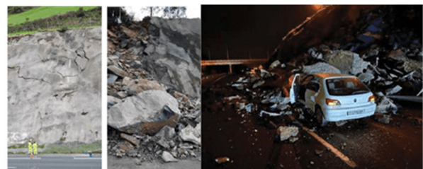
Figure 8. Slope detachment. Initial situation. Removal of material to provide traffic.
