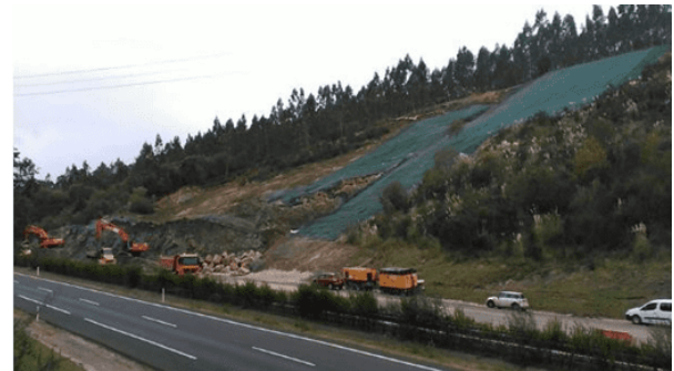
Figure 7. . Slope detachment. Removal of material to provide traffic on the left lane.
