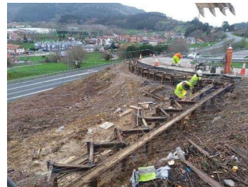
Figure 16. Welding the rails of the rail jacking to contain the CA-502 platform.
