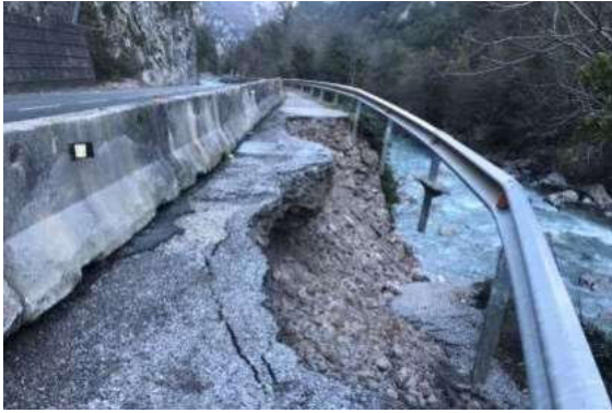
Figure 9. Collapse of wall N-621 pk 161.950
