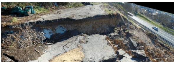
Figure 5. N-629. Slope landslide. Initial situation. Road platform at the head of the slope.
