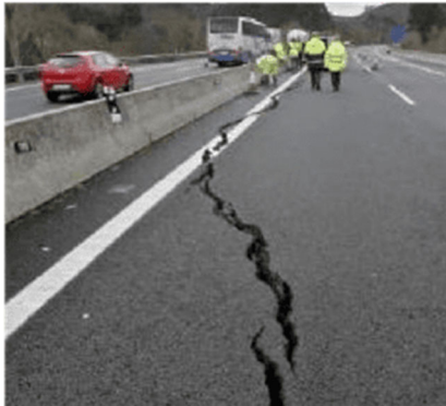
Figure 3. Cracking the carriageway with a 100 cm drop on the A-8 motorway, Liendo.
