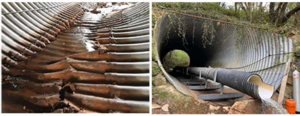
Figure 25. N-623 KP 103+800. ARMCO pipe collapse. Initial situation and river diversion
