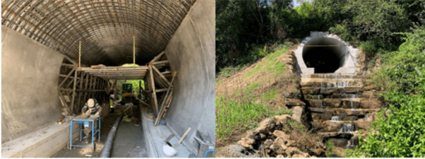
Figure 26. N-623 PK 103+800. ARMCO pipe collapse. Formwork and exit with natural projections.
