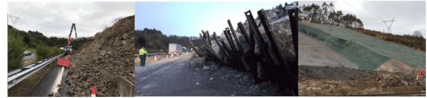
Figure 6. Landslide occupying the entire left-hand carriageway of the dual carriageway. Morning of 11 November 2017. Left lane enabled traffic and constant pushing of the landslide bending the driven lanes. Laying of geogrid, triple twist mesh and cable nets.
