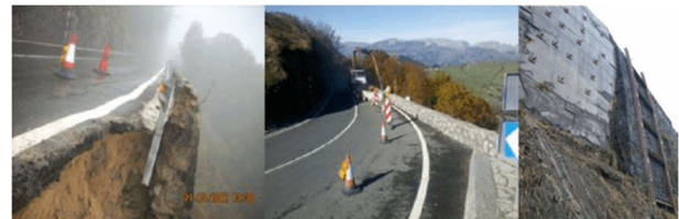
Figure 23. Sinking of the N-629 roadbed caused by heavy rains, provisional signalling and reinforcement of the masonry wall.
