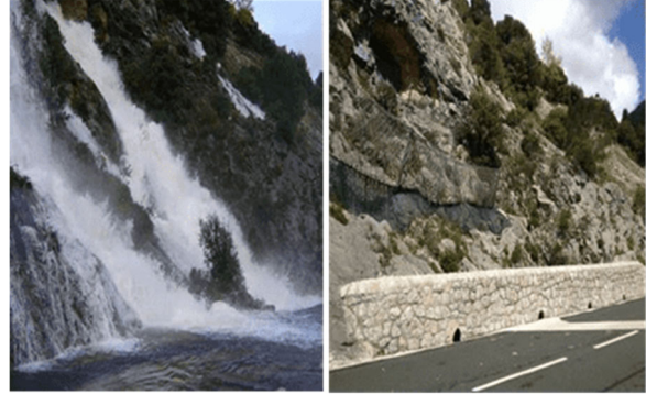
Figure 11. Situation of PK 158.140 MI caused by heavy rains.
