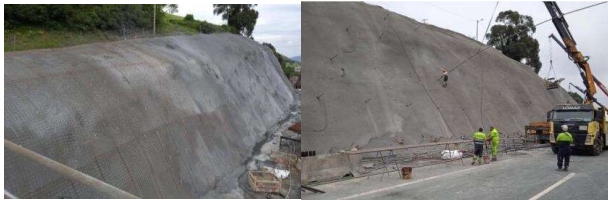
Figure 19. Stabilisation of the slope of the A-8 motorway (E-70). Placement of electrowelded mesh and anchors.
