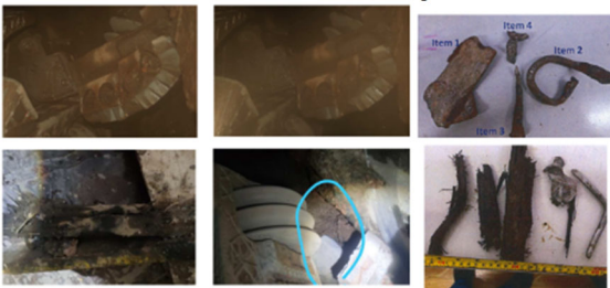
Figure 12. MTBM blockage and obstruction
