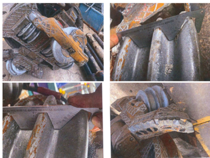
Figure 13. Cutter head Condition after 1 st row of MTBM.
