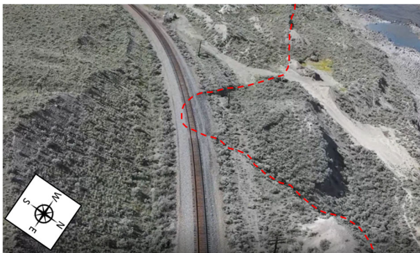
Figure 2. Active landslide slump block impacting 30 m of track.
