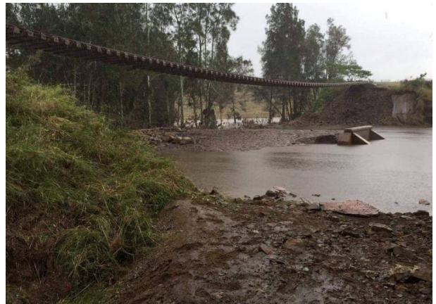
Figure 6. Photograph of the Tocal rail embankment washout taken at the bottom of embankment.
