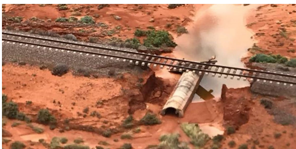
Figure 1. Flood damage to the Trans-Australian railway line near Tarcoola, South Australia, Jan 2022.
