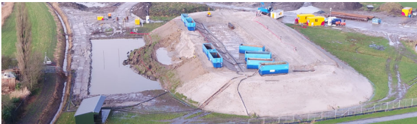
Figure 9. Aerial view of the Eemdijk test embankment with the failed slope of the GD on the left side (Lengkeek, 2022).
