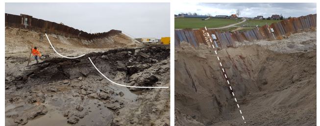
Figure 10. Left Side view of the SPD failure mode after draining the ditch, with clear indication of the exit point of the slip circle. Right Top/back view of the sheet piles after failure and local excavation, the dashed line indicates the inclination of the sheet pile. All interlocks of sheet piles are still intact.
