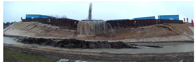
Figure 9. Photo at the moment of failure (16:00 hr.), showing the pushed-up slip circle, the sheet pile deflection and overtopping.
