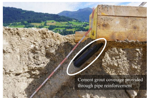
Figure 4. Improved cement grout coverage of the steel bar achieved through pipe reinforcement.
