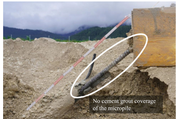
Figure 3. No cement grout coverage at the transition to the concrete foundation.
