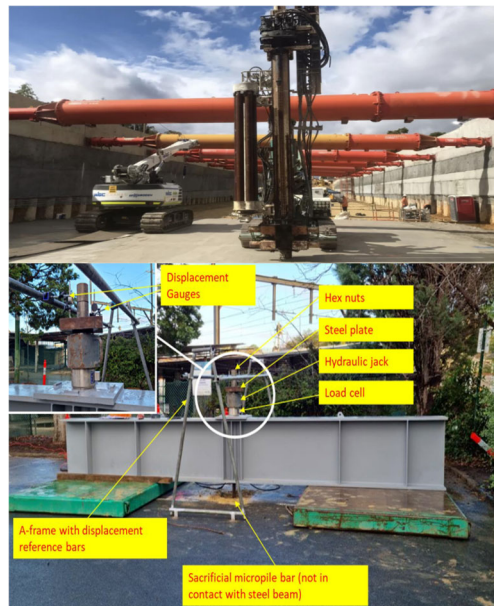
Figure 9. Micropile drilling rig at base of excavation level and pull out testing setup on sacrificial micropiles.
