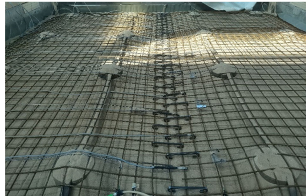
Figure 2. The large-scale test set-up showing the deformed steel mesh during excavation after test performance. Some of the 16 piles with a diameter of 225 mm and instrumentation are visible (2023, TU Darmstadt Geotechnical Test Pit facility)
