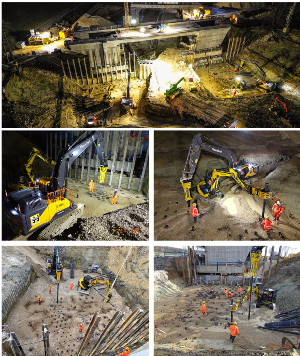
Figure 12. Installation of the DIPs for the ground improvement (courtesy of Carl Heuchel GmbH & Co. KG)
