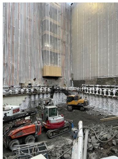
Figure 4. The image shows excavation work in progress, milling of frozen soil inside sheet piling and insulation in Area 1. Above the Berlin shoring, the feed lines and connection to the freezing pipes are visible.
