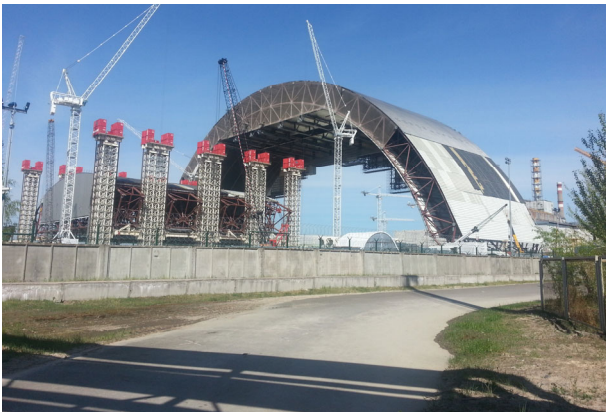
Figure 3. First section of the vault placed in the transfer zone and the second one's beginning
