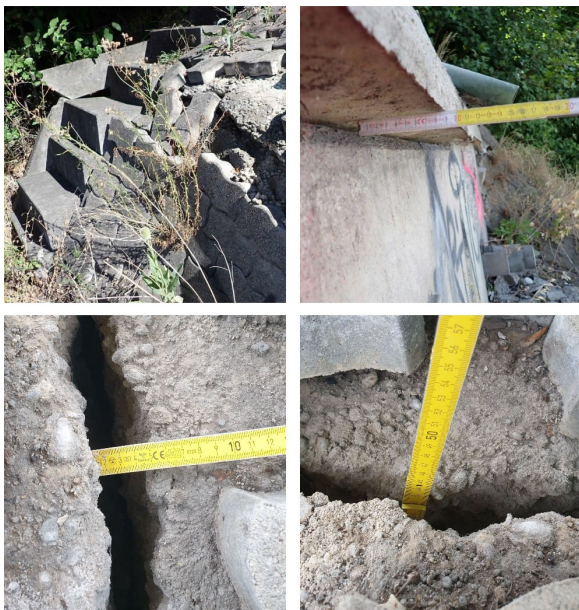
Figure 4. Deformation of the steps and crack measures.
