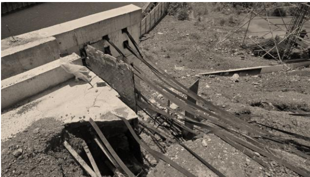
Figure 3. Exposed geosynthetic strips of the MSE wall due to erosion.
