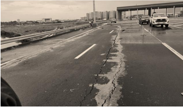
Figure 1. Pavement cracks with differential settlement.
