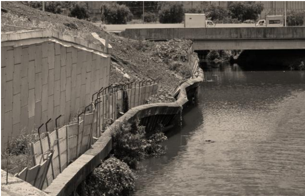
Figure 2. Tilting of sheet pile walls.
