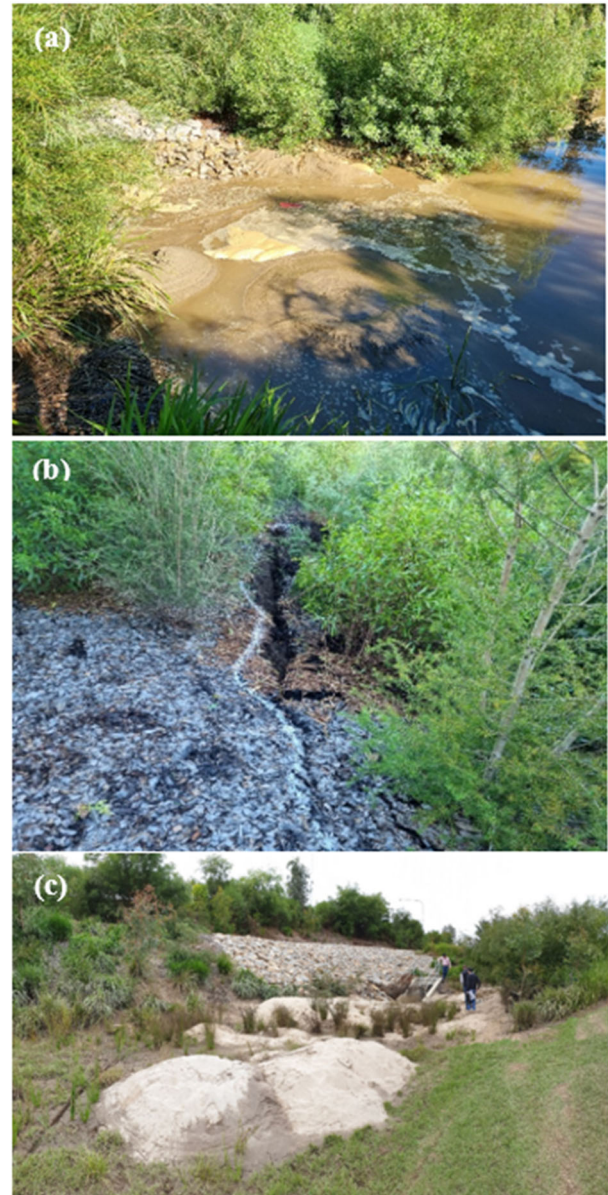
Figure 3. Observations of (a) water ingress and sand boiling in basin; (b) tension cracks on basin batter on 24 March 2021; and (c) sand deposited on basin floor after water subsided.
