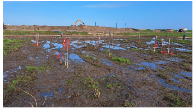
Figure 11. Photo of full-scale test with pore water pressure meters at the front.
