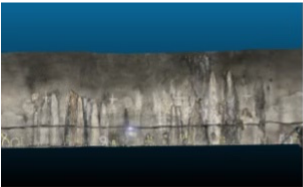
Figure 5. Figure 1. Zoomed detail of water leakage detected in the tunnel lining.
