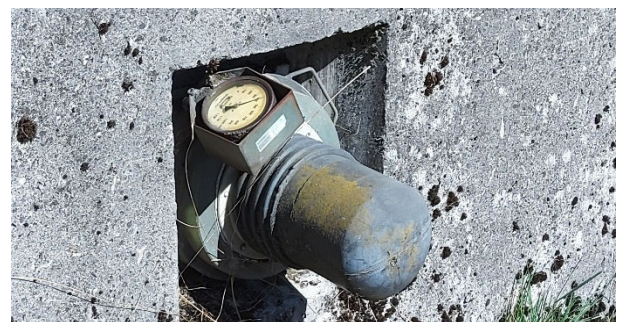
Figure 3. Hydraulic pressure cell with an analogue gauge used as an anchor load measurement device.
