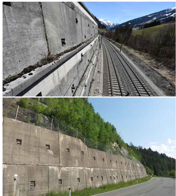
Figure 1. Examples for anchored retaining structures, diagonally anchored element wall (top), segmented anchor wall (bottom).
