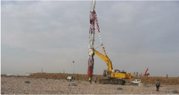
Figure 9. Strip vertical drains and preloading in new quay esplanade of Barcelona Port.
