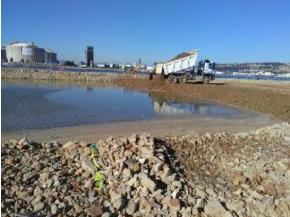
Figure 13. CDW aggregate (750.000m 3 ) backfilling Adossat quay wall. APB (2019). Unpublished image. Reproduced with permission.
