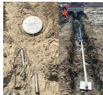
Figure 5. Circular pressure cells (D = 30 cm) placed on CMC (left) and Inclinometer installation in the LTP (right)
