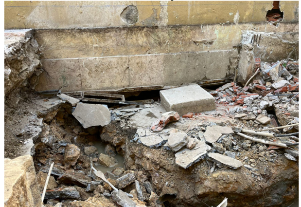
Figure 22. Floor collapse and unfooted Wall.
