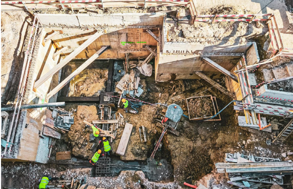
Figure 21. Execution of the definitive foundations as proposed for the stabilization of the deformations.
