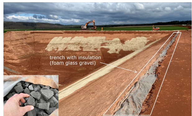
Figure 7. Execution of the edge insulation proposed based on modelling results. Source: Ramboll.
