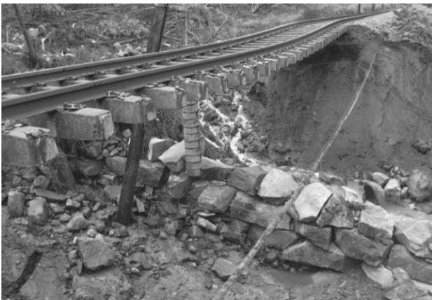
Figure 1. Example of total destruction of embankment around culvert near Ål, Bergensbanen railway line (Oslo to Bergen).
