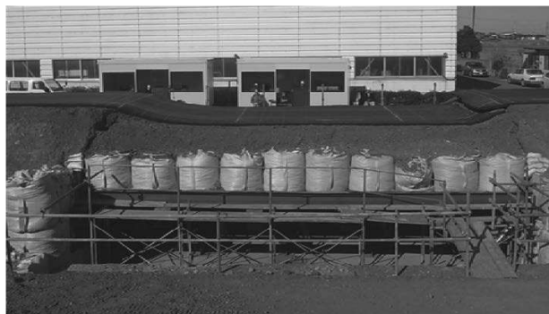
(1) Testing result after 550mm differential settlement
