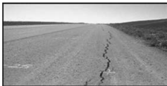
Figure 2. Longitudinal cracks near the edge of pavement
