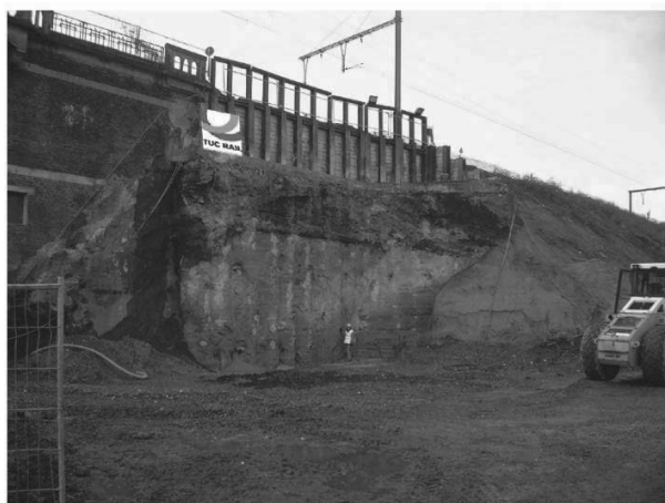
Figure 7. Photo of retaining wall after final excavation phase, after backfill for piling rig
