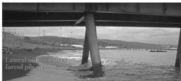
Figure 1. Bending and displacement of pile foundation at Puerto de Coronel Muelle wharf.
