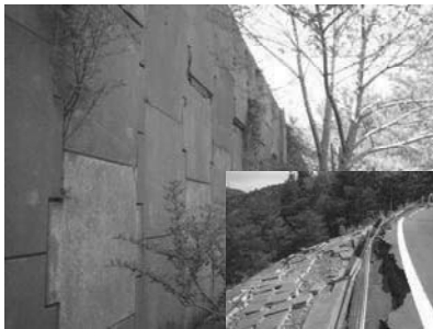
Photo 3. Collapse of embankment and the deformation of wall's surface
