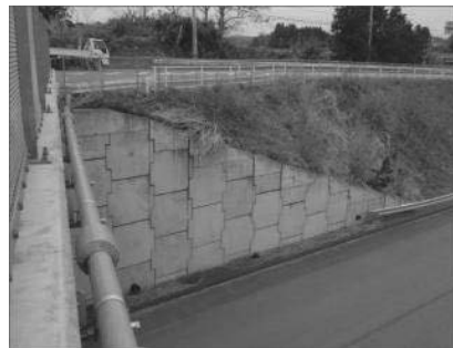
Photo 2. Wall in the area of seismic intensity 7 (Rank I)
