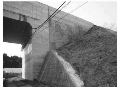
Photo 1. Wall in the area of seismic intensity upper 7 (Rank II)
