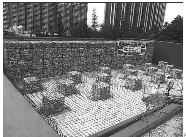
Figure 1. Array of baffles installed in front of a rigid barrier in Lantau Island, Hong Kong
