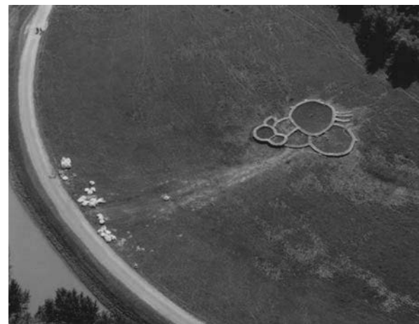
Figure 3. Piping (soil boiling) far away from the dyke, and stabilizing measures to reduce the hydraulic gradient (photo: L. Nagy).
