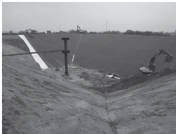
Figure 6. Photo of pit during completion of excavation and laying out of the membrane in progress. The tower in the centre of the photo is a 16 m tall water in- and outlet for the operational phase of the PTES.
