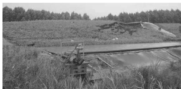
Figure 4. West dike close before failure.
