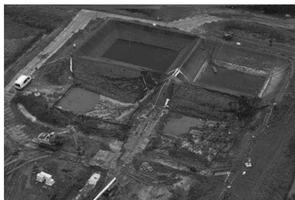
Figure 5. West and East dikes after failure.
