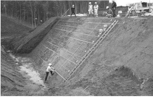
Figure 2 Field test setup
