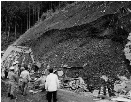
Figure 1 Typical example of labor accident during slope cutting works
